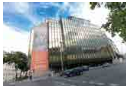
The BUWOG Group is working together with the "BauKarrusell" cooperation network and the "Harvest Map" recycling platform on the dismantling of the property at Rathausstrasse 1 in Vienna.
